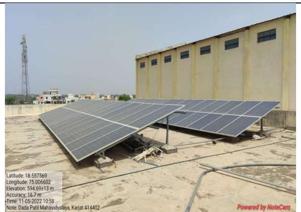
Wheeling to the grid
