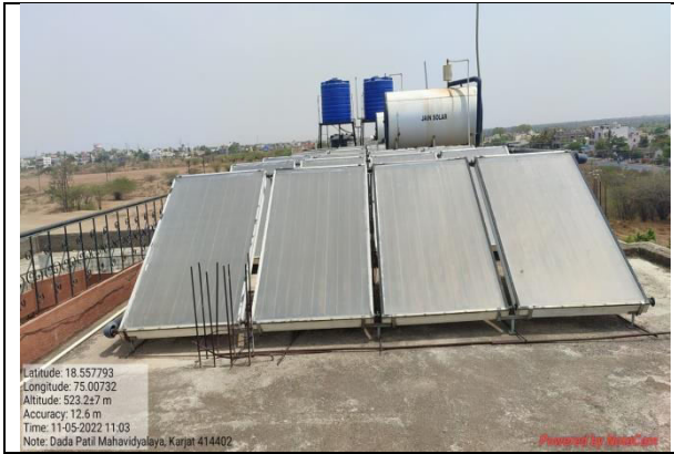
Solar Energy Plant
